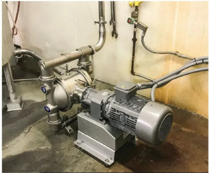
Image 1. An EODD pump in an installation (Images courtesy of Graco Inc.)
